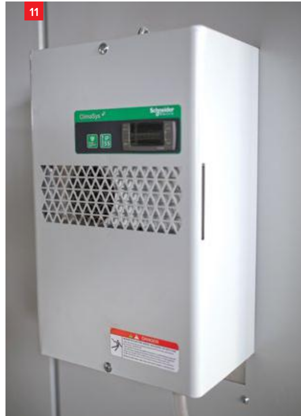
11 Elektrik Panosu Klima Sistemi Electrical Panel Air Conditioning System
